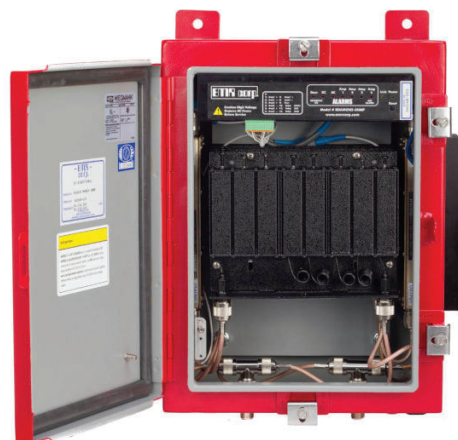
EMR BDA System with BDAMON2 installed.
